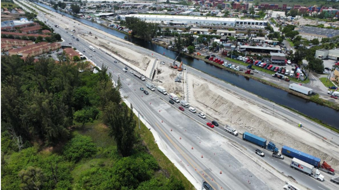
Aerial photo of Okeechobee Rd east of NW 116 Way showing the second level overpass under construction.
