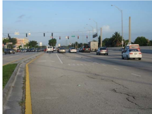
View of pavement conditions. The study corridors are in fair condition. Milling and resurfacing is recommended along both, SW 87 th and SW 8 th Street
