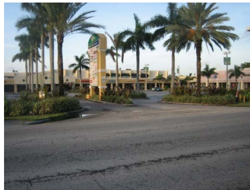
View of the SW 8 th Street corridor east of SW 87 th Avenue. From field observations it can be determined that the pavement is in need of milling and resurfacing
