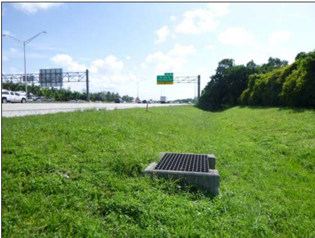
Figure 11 – 4: Berms and Ditches within the Archaeological APE on the Eastern I-95 ROW near the NE 203 rd Street Interchange, Facing Northeast
