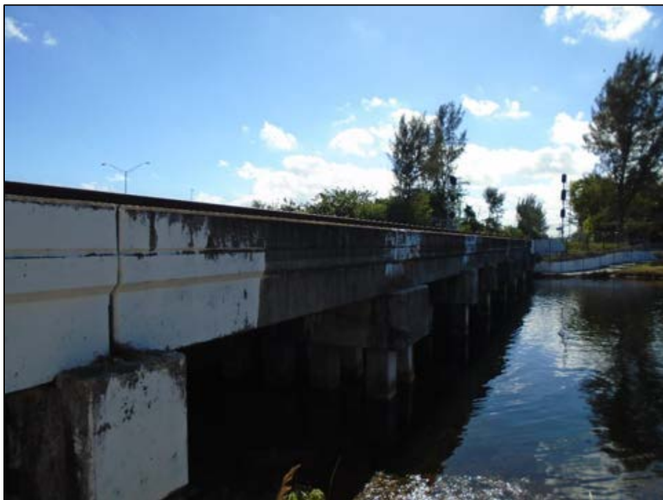
Figure 11 – 15: CSX Railroad (8DA10753) over Snake Creek Canal, Bridge Substructure, Determined National Register-Eligible, facing South
