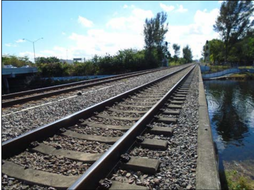
Figure 11 – 14: CSX Railroad (8DA10753) over Snake Creek Canal, Determined National Register-Eligible, facing Southwest
