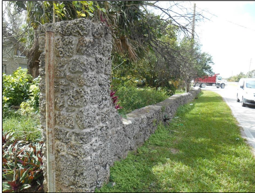
Figure 3-2: Oolitic limestone exterior wall, located at the northeastern corner of the National Register–eligible and locally designated Talbott Estate (8DA2789), facing west
