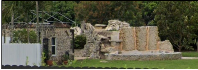
Figure 3-19: Southwestern outbuilding on the property containing the National Register-eligible building at 20000 SW 137th Avenue (8DA20713). This outbuilding is in a ruinous state. March 2021 Google Streetview photograph, facing southwest
