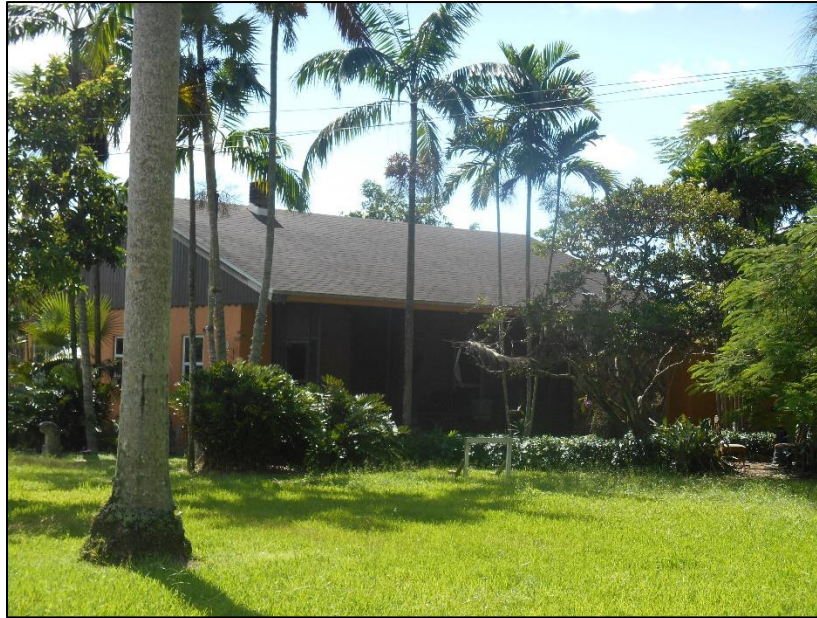
Figure 3-8: Northwestern corner of the cottage outbuilding south of the converted shed on the National Register–eligible and locally designated Talbott Estate (8DA2789), facing southeast
