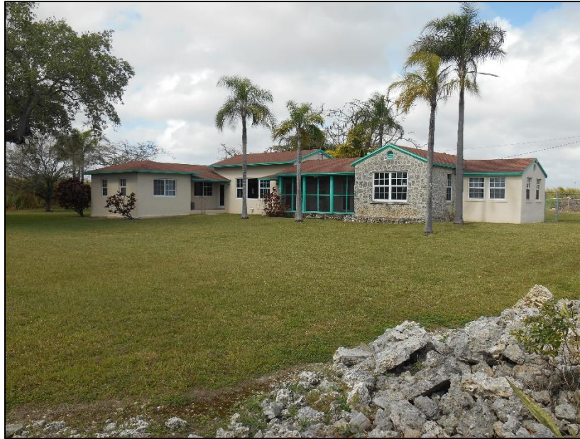
Figure 3-10: Southern elevation of the National Register–eligible MacDonnell Residence (8DA20712), with a damaged segment of the parcel’s oolitic limestone wall in the foreground, facing northwest
