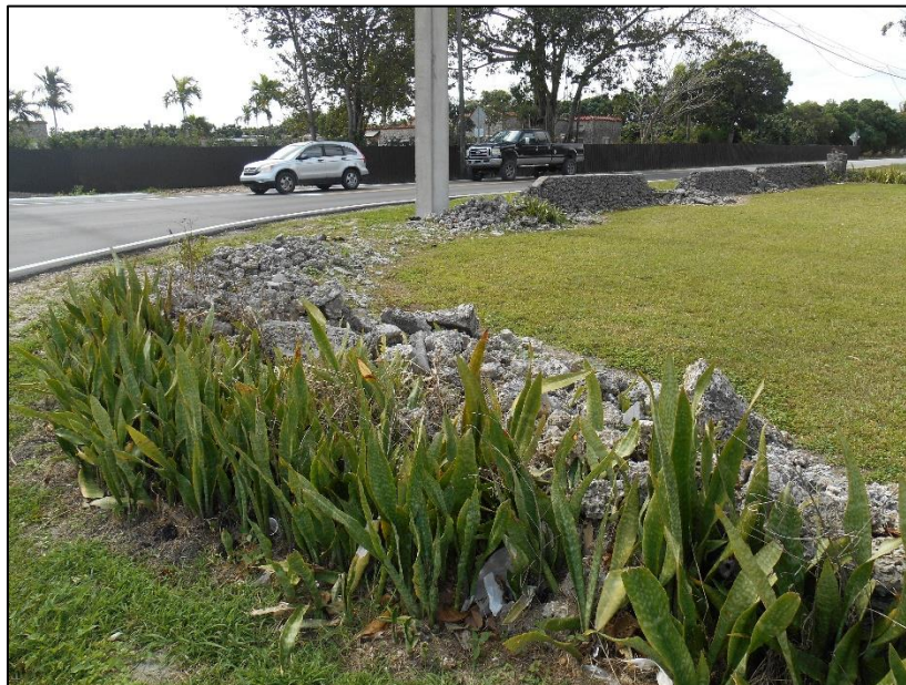
Figure 3-13: Damaged segment of oolitic limestone exterior wall, located at the southwestern corner of the National Register–eligible MacDonell Residence (8DA20712), facing northeast
