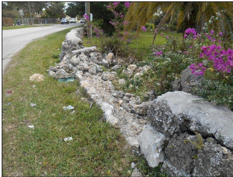
Figure 3-3: Damaged segment of oolitic limestone exterior wall, located at the northwestern corner of the National Register–eligible and locally designated Talbott Estate (8DA2789), at the intersection of SW 134th Avenue/Talbot Road and SW 200th Street/Quail Roost Drive, facing east
