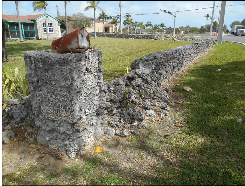
Figure 3-12: Damaged segment of oolitic limestone exterior wall, located at the southwestern corner of the National Register–eligible MacDonell Residence (8DA20712), facing northeast
